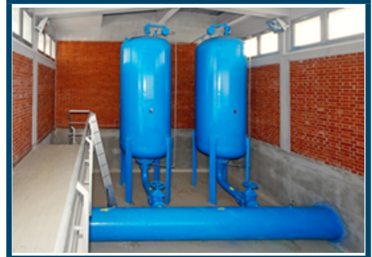
Figure 2 Two vertical air receivers
