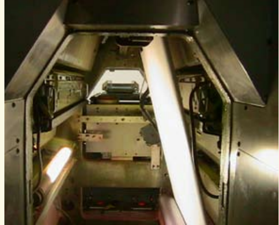
Printing press interior showing limited space. (Turbos are on either side). Hatch at rear is visible.
