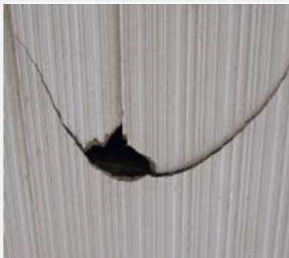
Figure 5 Examples of sharply broken edges on asbestos cement sheeting
