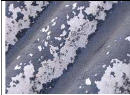
Friable asbestos roof cladding (friable)
