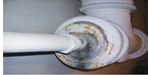
Amosite and chrysotile packing on a water pipe (friable)
