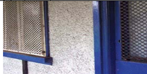
Chrysotile pebble dash exterior wall coating (non-friable)
