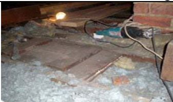
Friable asbestos debris (friable)
