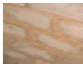
Non-friable - Asbestos bricks
