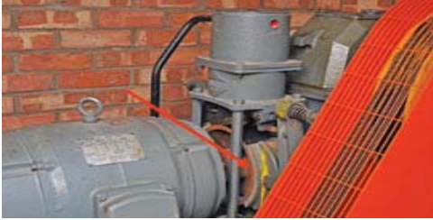
Asbestos brake lining on output shaft of AC motor (friable)
