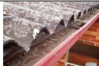
AC moulding gutter (friable)
