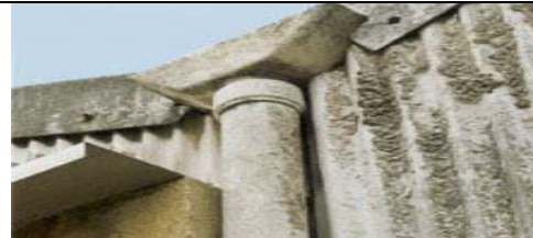
AC downpipe (friable)
