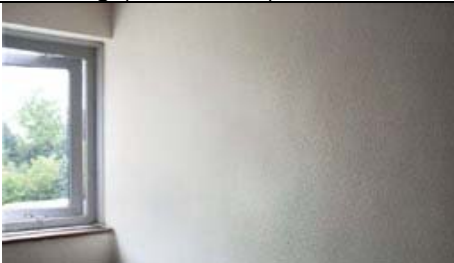
Wall plasters containing asbestos (non-friable)
