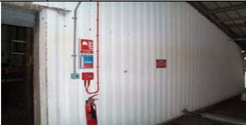
Asbestos bitumen coating under metal cladding (non-friable)
